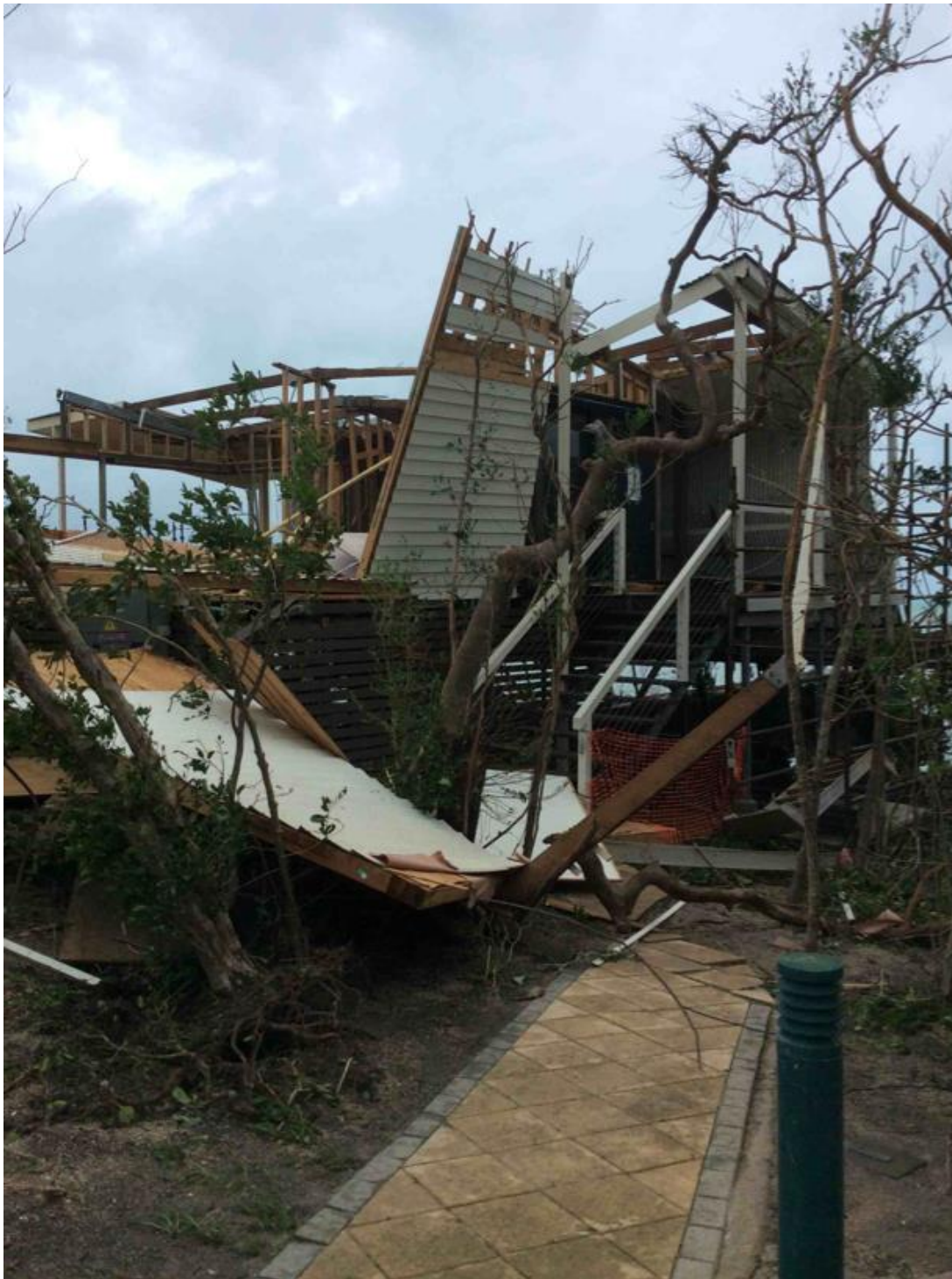
Figure 16. Building damage on Lizard Island. Photo supplied via Queensland Fire and Emergency Services (QFES).
