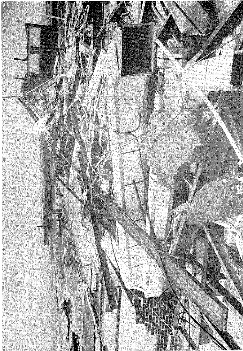
Part of the damage to the Port Hedland District Hospital.
