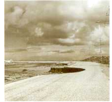
Erosion which occurred during Severe Tropical Cyclone Vance near Exmouth, 1999.
