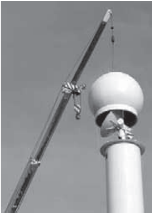
Final stages of the installation of the new radar at Gove (Northern Territory).
