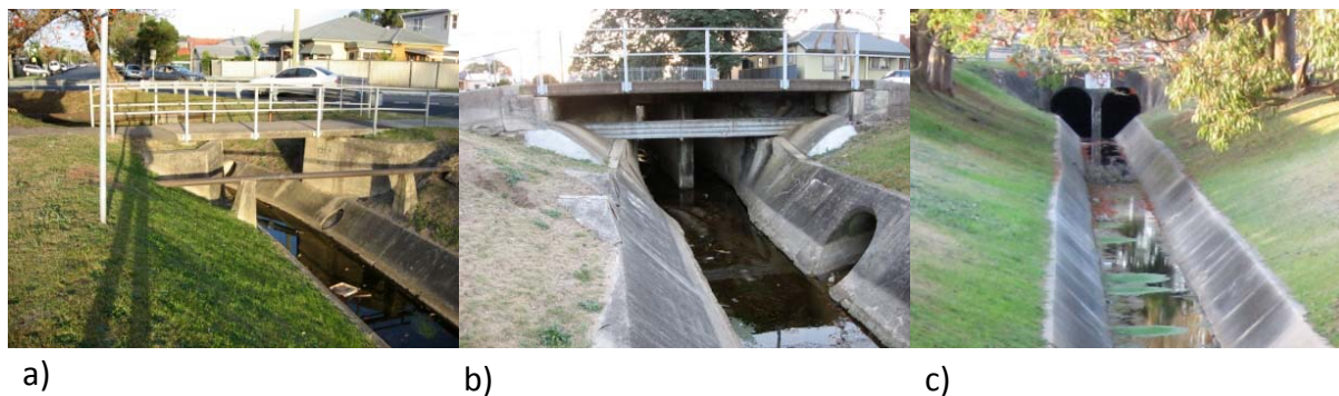
Figure 5 Stormwater system features that capture debris (a) low pipes below ground elevation, (b) pipes, telecommunications, and in-stream piers, and (c) open channel to culvert transitions.
